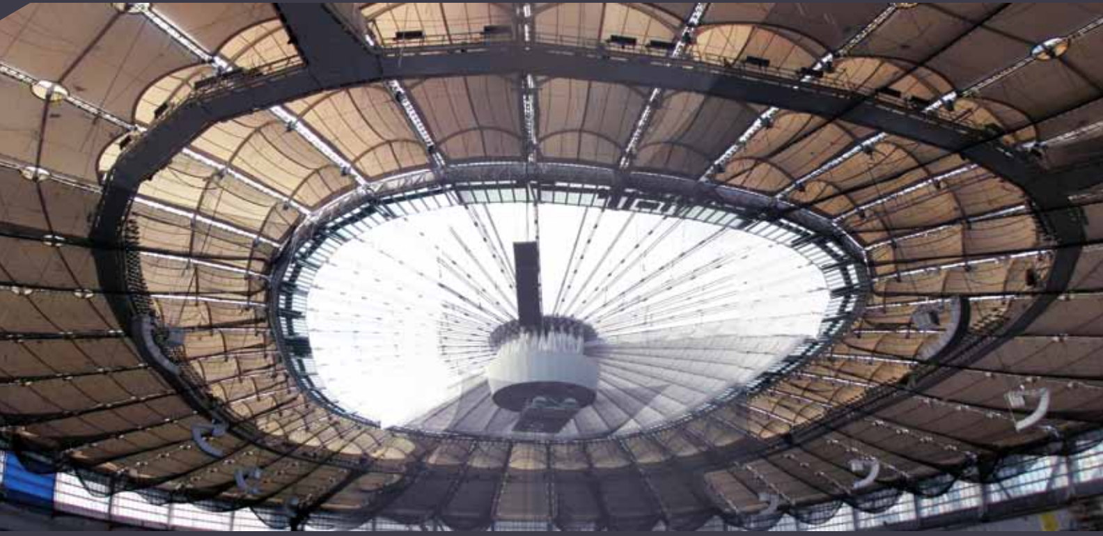
▲ PHOTO: 18,000 TONS OF STEEL AND 76,000 SQUARE METERS OF FABRIC WERE USED IN THE CONSTRUCTION OF THE NEW RETRACTABLE ROOF.
